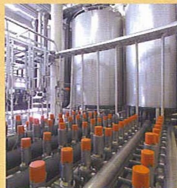
ABB drives have helped Valio to achieve high levels of hygiene at its cheese plant in Joensuu, Finland
